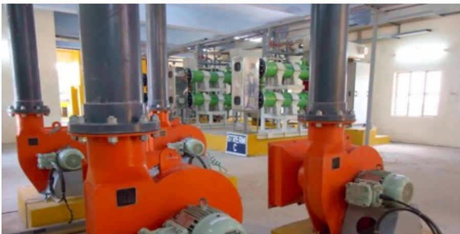
RT CHLOR-BCT Modular system Hydrogen Dilution Blowers
