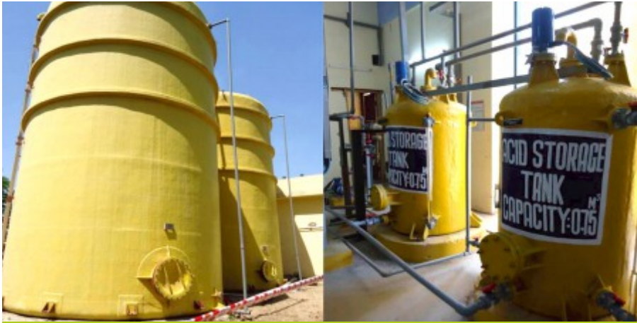
RT CHLOR-BCT Modular system Hypochlorite Storage tanks and Acid Cleaning system
