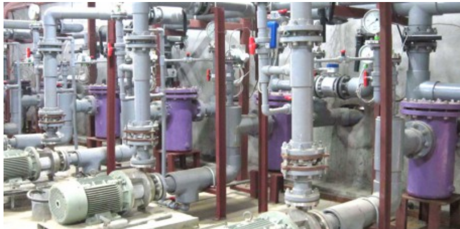
RT CHLOR-BCT Modular system Dosing Pumps Assembly
