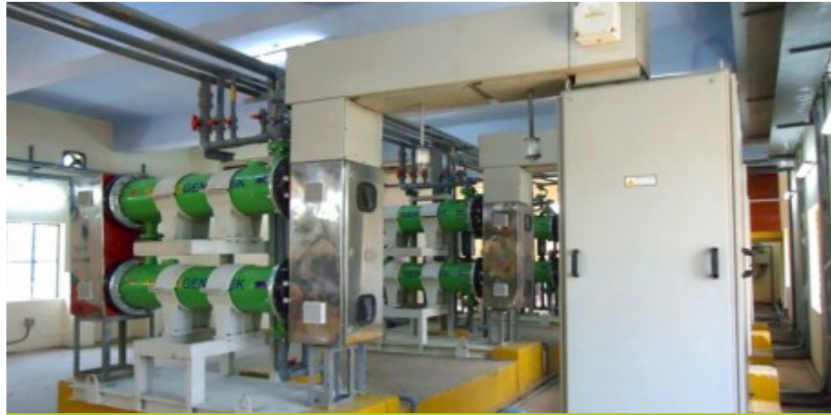
RT CHLOR-BCT Modular system Electrolyser Assembly along DC power Bus-duct
